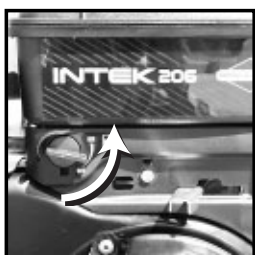
Fuel shut-off valve
